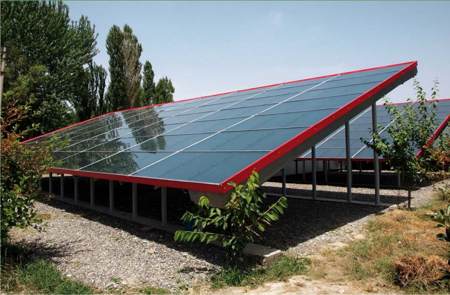
Solar air collector system in Uzbekistan.
