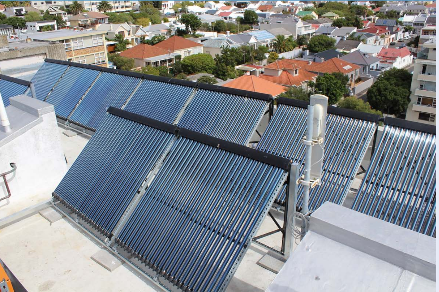
85 m 2 evacuated tubes at Centurion Building, CapeTown
