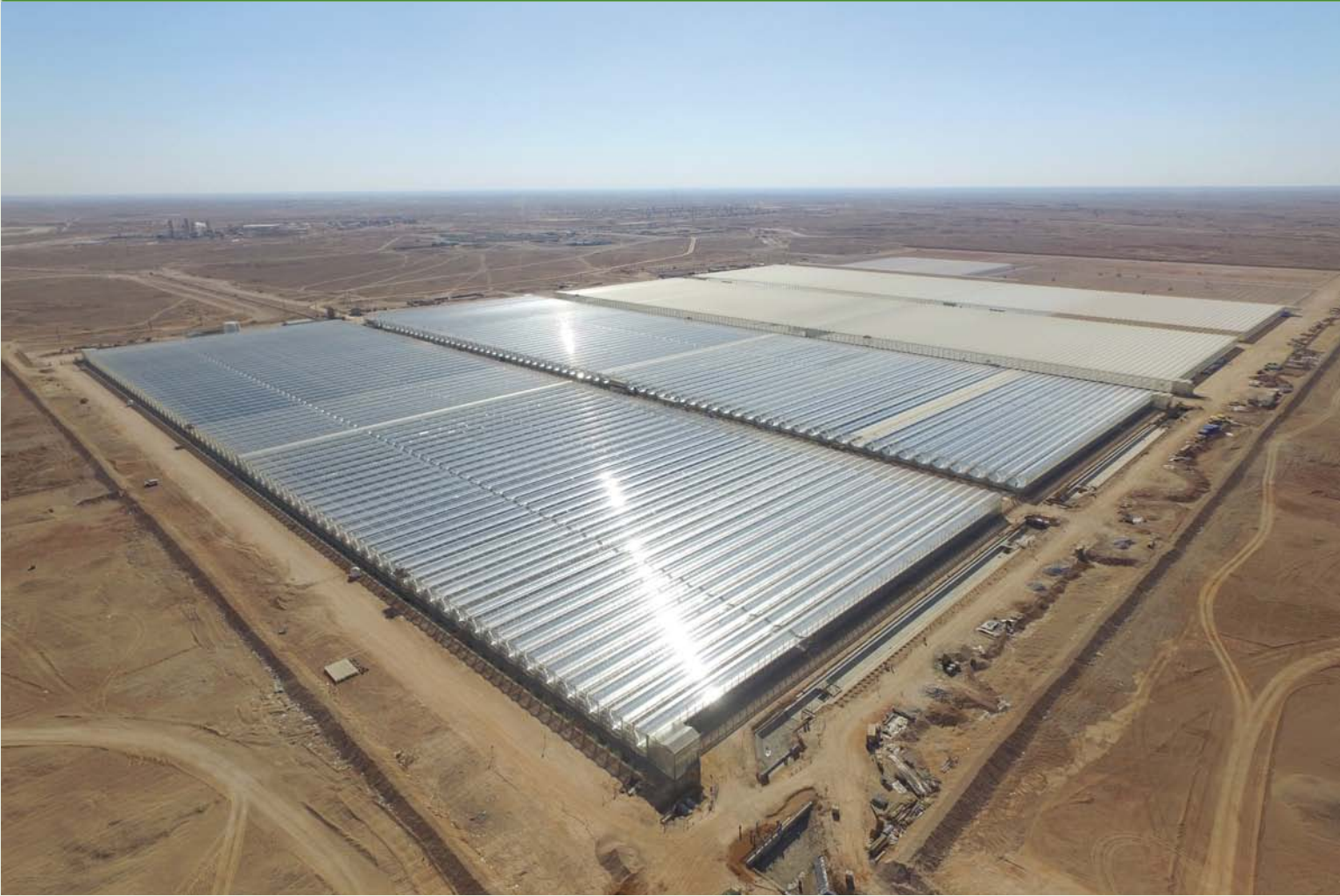
Four blocks of the Miraah solar plant with a total capacity of 100 MW th .
