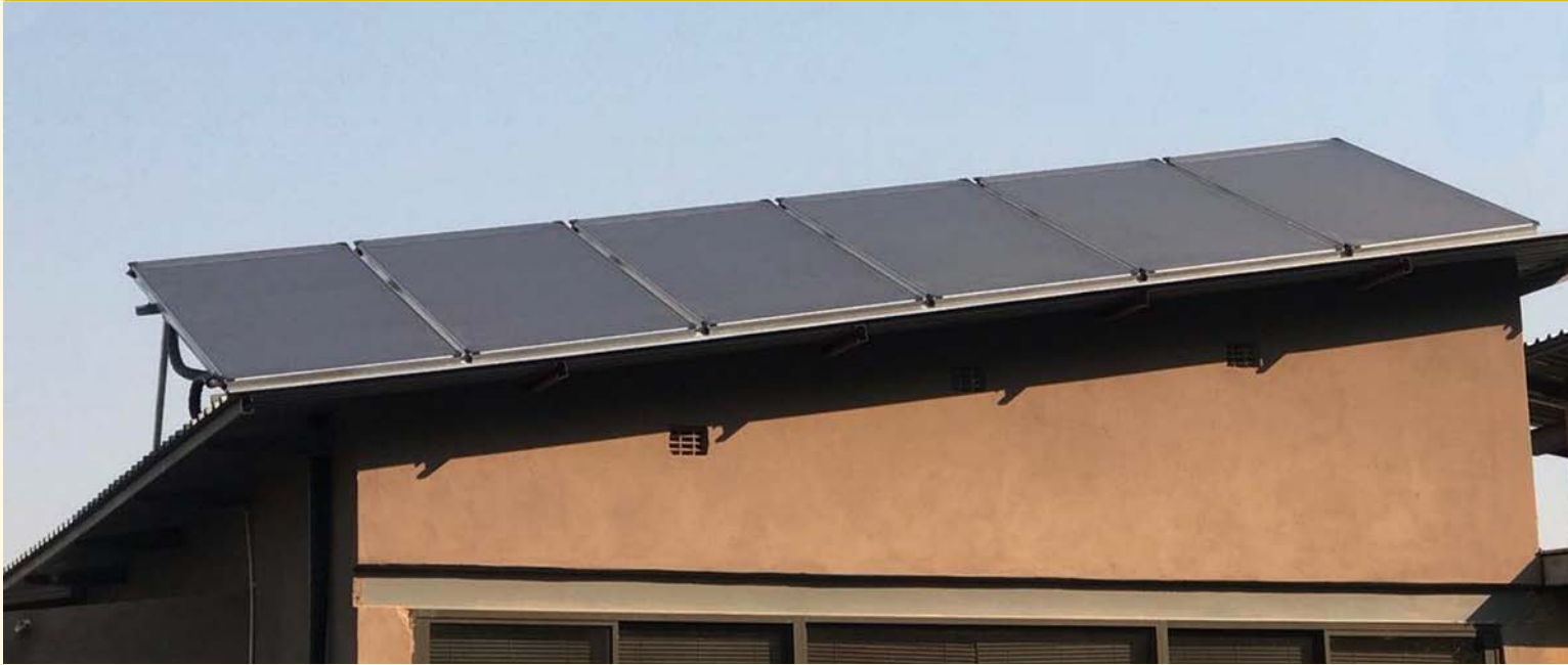
14 m 2 flat plate collectors at Thatch View Lodge, South Africa
