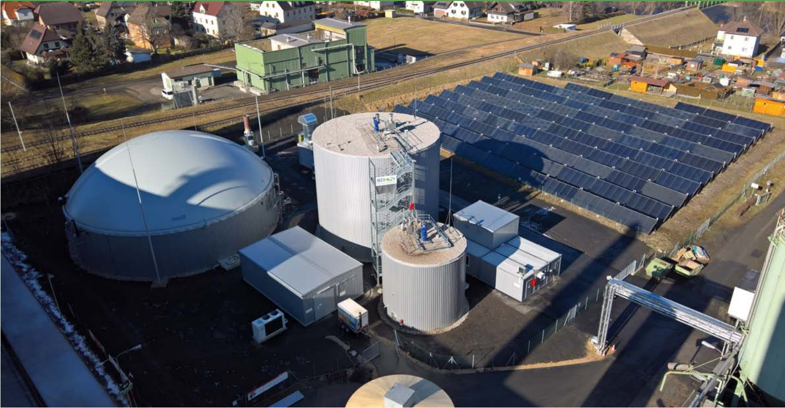
1 MW th solar process heat plant at the Goess Brewery in Austria.
