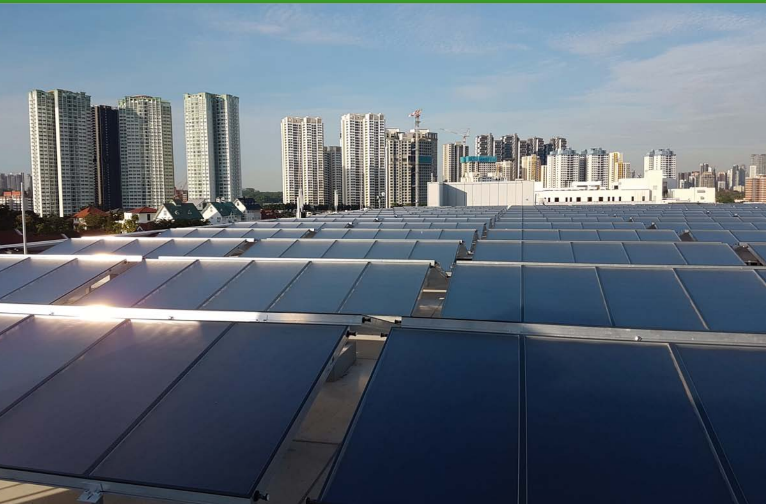
2,472 m 2 solar cooling system at IKEA Singapore delivers 1,587 MWh for an 880 kW absorption chiller.
