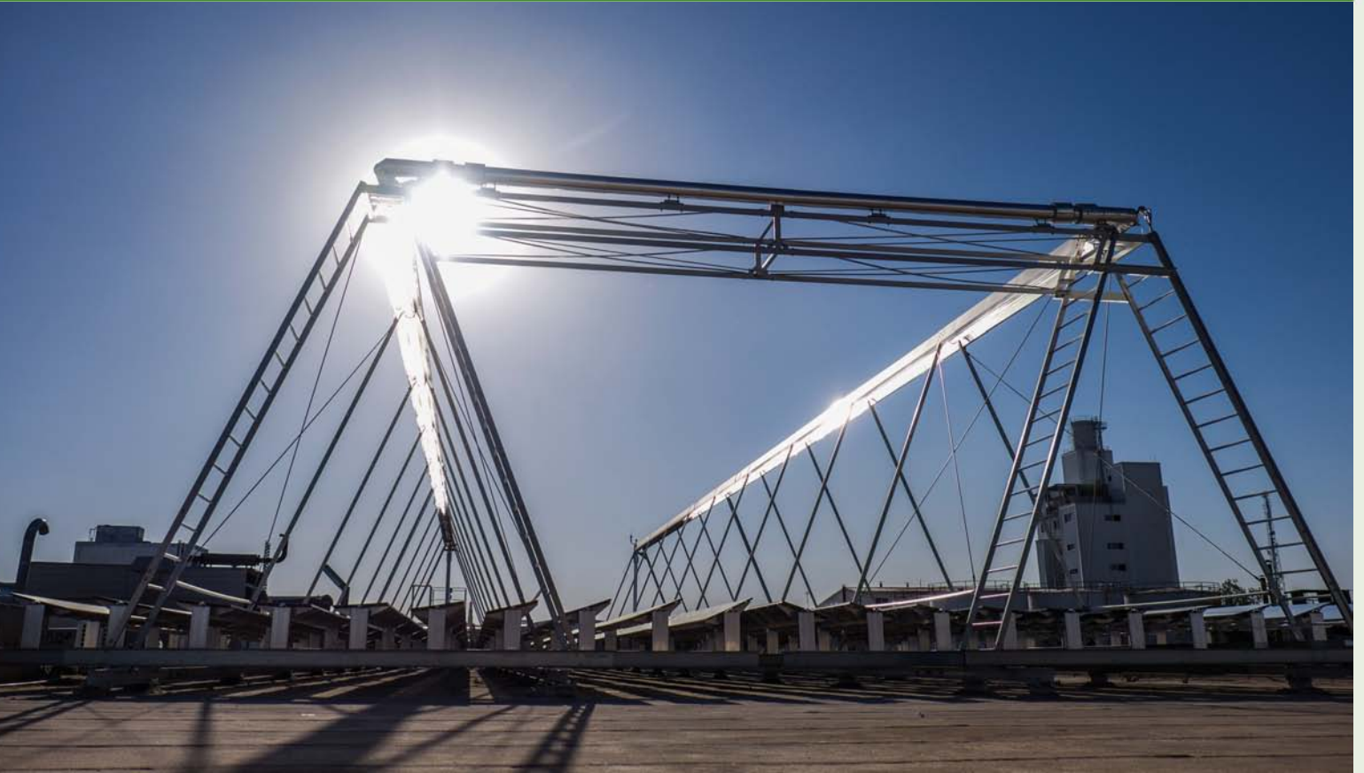
Fresnel collector field for direct steam generation in Jordan.
