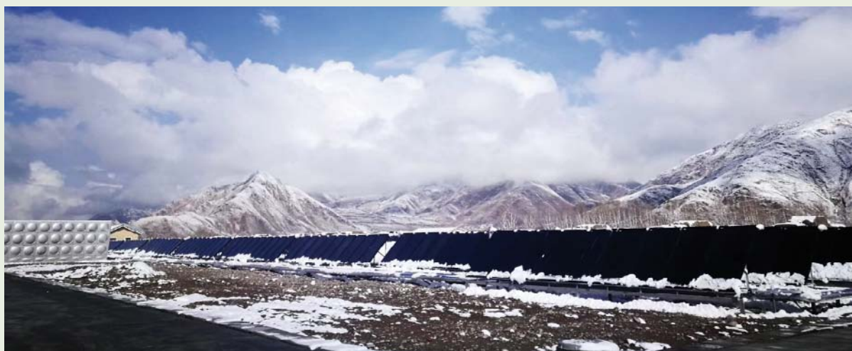
3,200 m 2 solar space heating project in Lhasa, Tibet.
