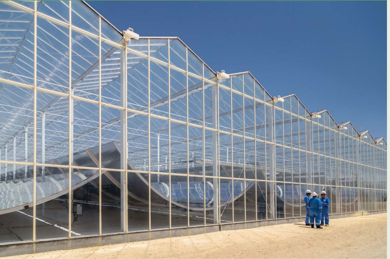
Indoor parabolic trough collectors at the Miraah plant in Oman.
