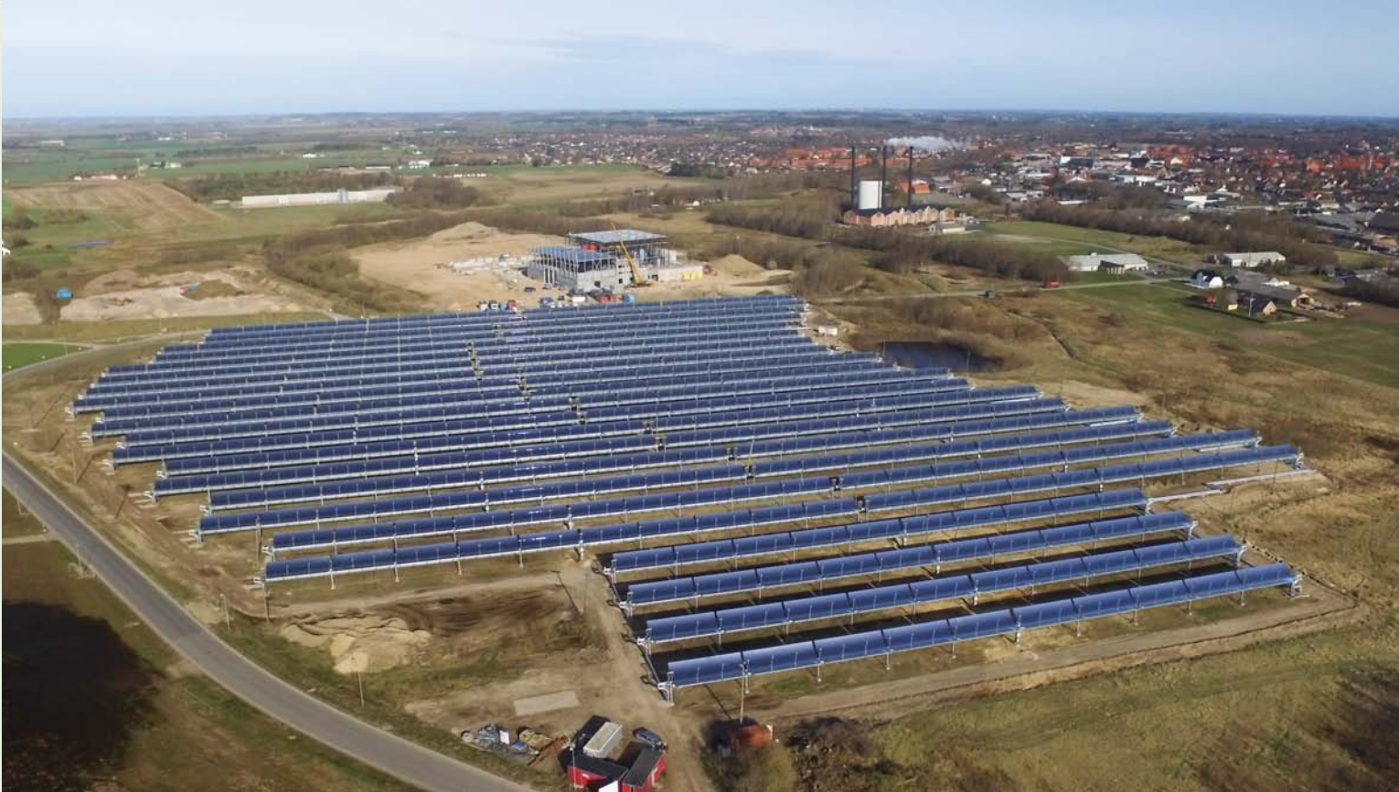
Parabolic trough collector field in Brønderslev, Denmark with an installed capacity of 16.6 MW th supplies not only heat to the district heating network, but also to power production as an add-on to a biomass-fuelled ORC system.
