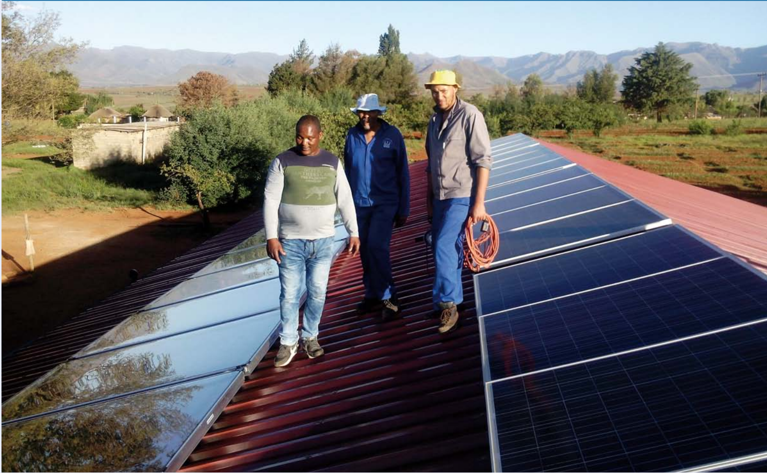
30 m 2 flat plate collectors at Pitseng Highschool, Lesotho
